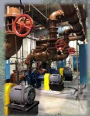
Secondary Treatment Pumps
