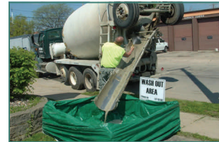
Vinyl washout container
