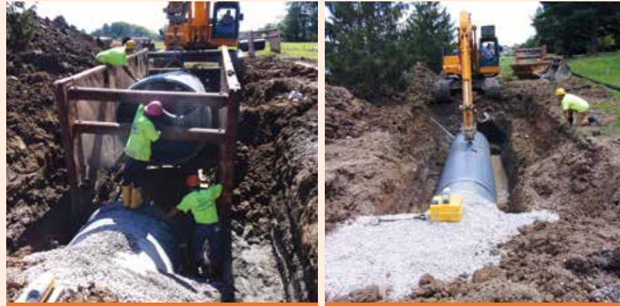
Replaced the existing 72" corrugated metal pipe storm sewer with a new 60" storm sewer in an easement on the south side of Roxbury School.
